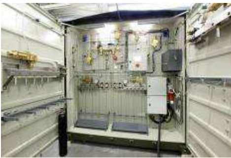
Cylinders filling ramp
