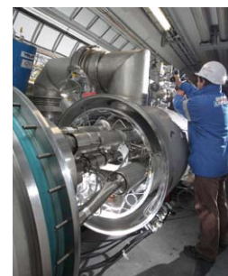
Cryogenic transfer lines
